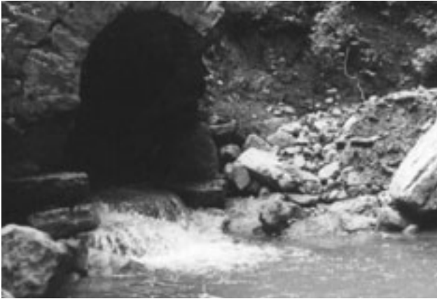
August weather hammered CPF trails. An access road had to be created to repair this collapsed stone arch.
